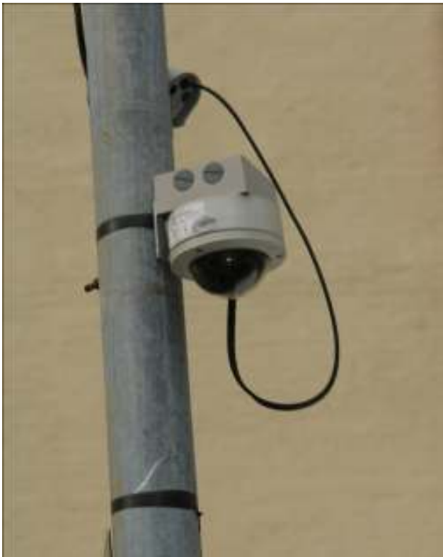
Figure 2: Installed Camera in the City of Pittsburgh
